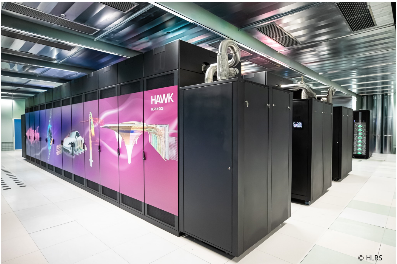
Hawk, the new supercomputer at the High-Performance Computing Centre (HLRS) in Stuttgart has over 720,000 cores and is almost four times faster than its predecessor.
